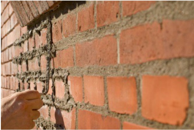
Professional workmanship when fixing cracks in foundation to match your current home
