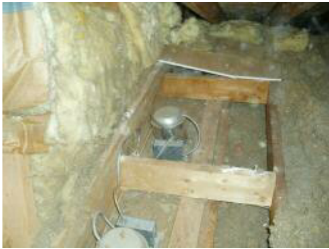
Replace no IC rated Recessed Lighting with new IC rated (IC Stands for Insulation Contact)
