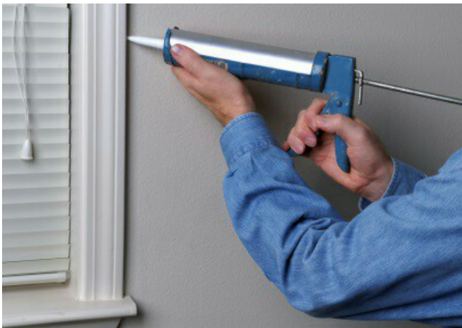
Caulk around windows
